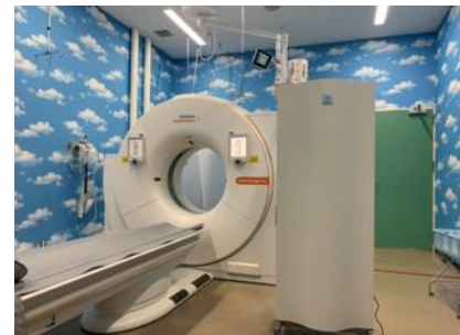
Figure 2: Genano 5250A air purifier in CT room
